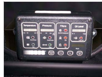
BCU Installed on Bracket
